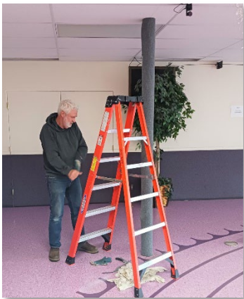
Above: Dan Andersen replaced the pole covers in the Social Hall in April.
