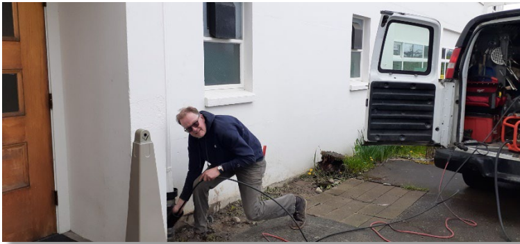
Dean Paulsen repaired a gutter drain line next to the main entrance in the lower parking lot.
