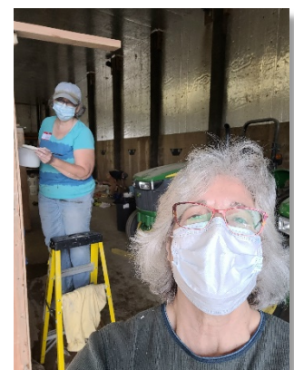
Betsy Loyer takes a break during the build for a selfie with Valorie Paulsen looking on!
